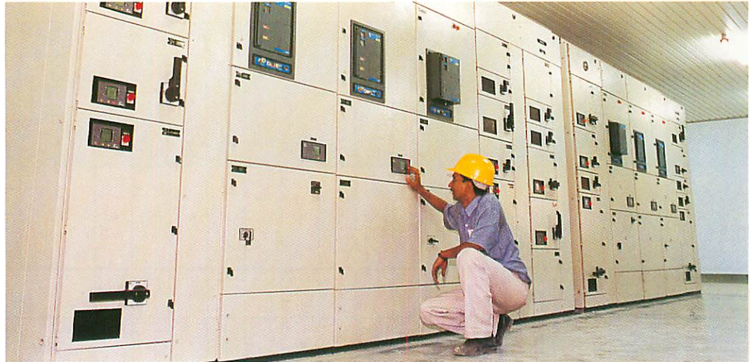
Larsen and Toubro (L&T) LV PCC Switchboard
