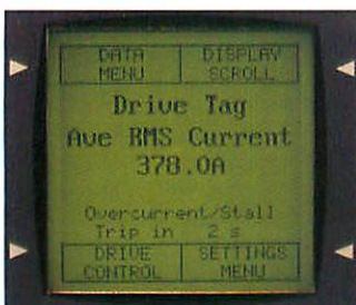
Timing out to trip on an Overcurrent condition
